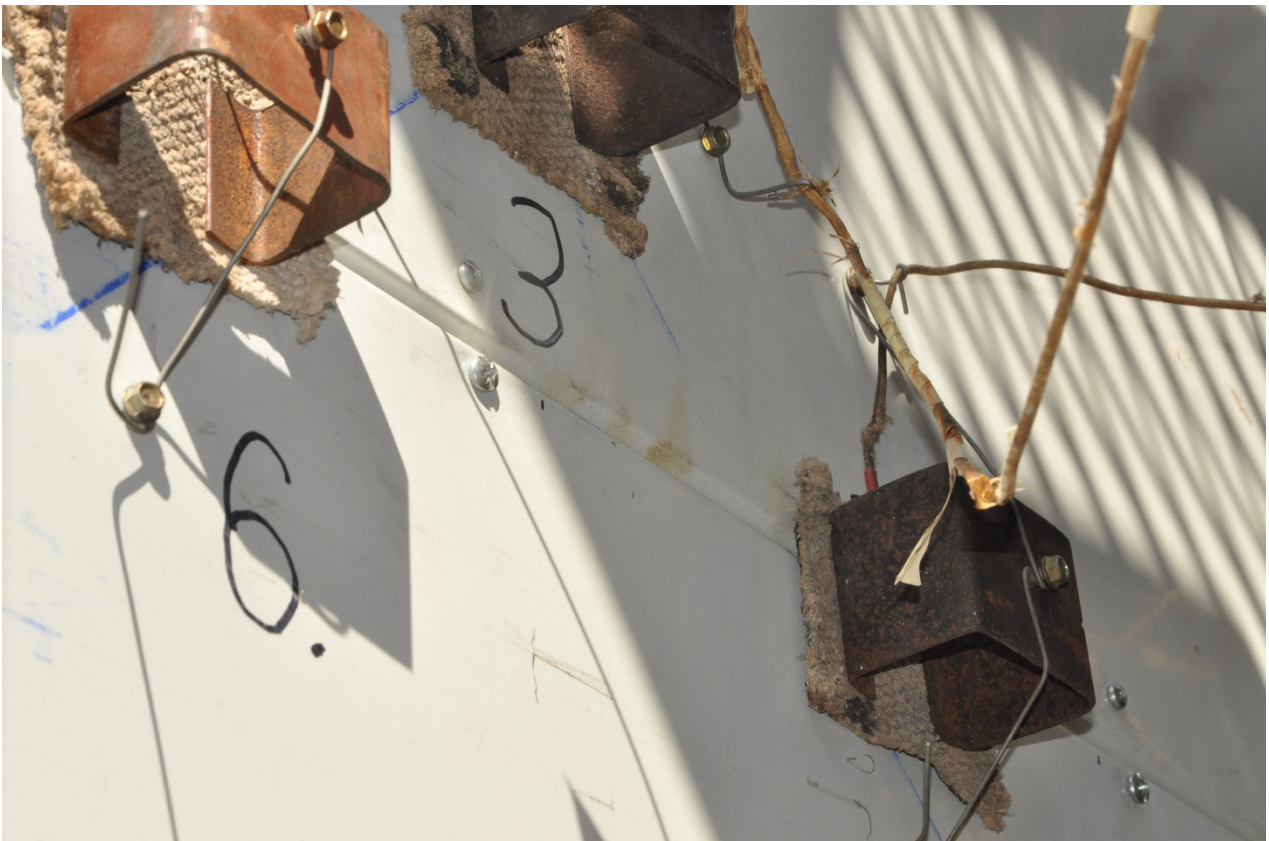
Figure 3.9: Discolouration on bottom joint
