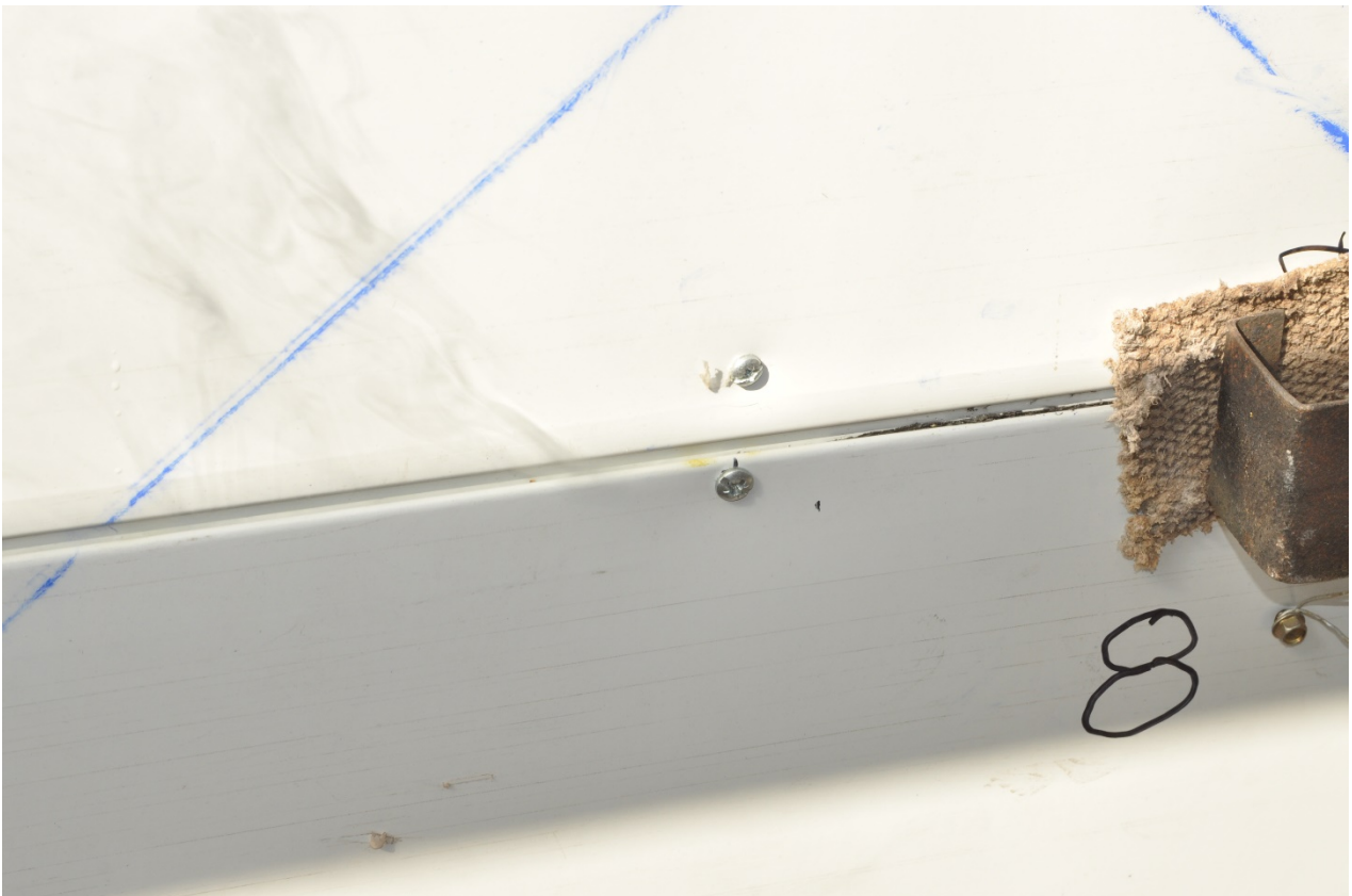
Figure 3.7: Smoke release from top joint
